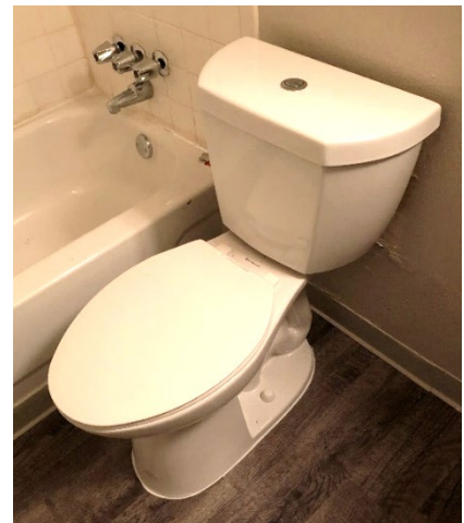
Ultra-high efficiency 0.8 gallons/flush 1
