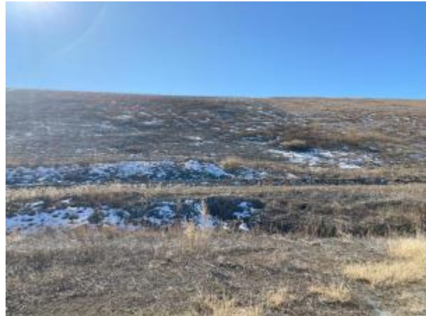
Photo No. 49, 12.03.2024 Observations
