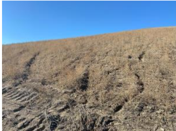
Photo No. 37, 12.03.2024 Observations
