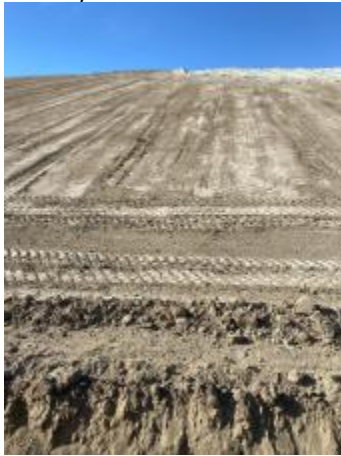
Photo No. 52, 12.17.2024 Observations
