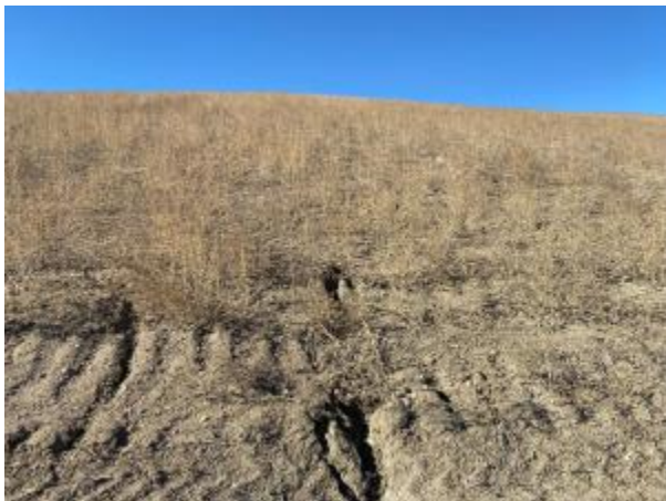
Photo No. 38, 12.03.2024 Observations
