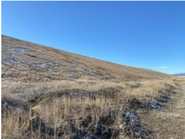
Photo No. 42, 12.03.2024 Observations
