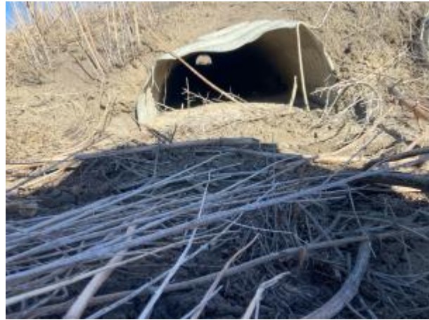
Photo No. 23, 12.03.2024 Observations
