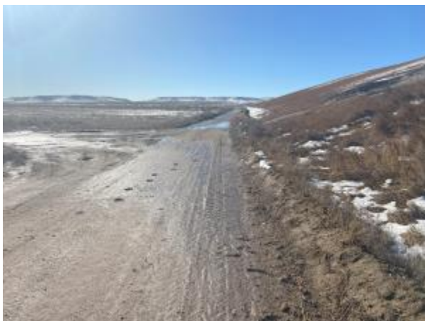
Photo No. 5, 11.13.2024 Observations
