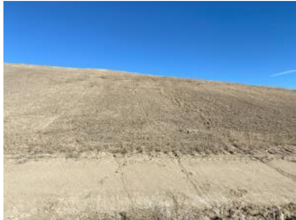
Photo No. 31, 12.03.2024 Observations
