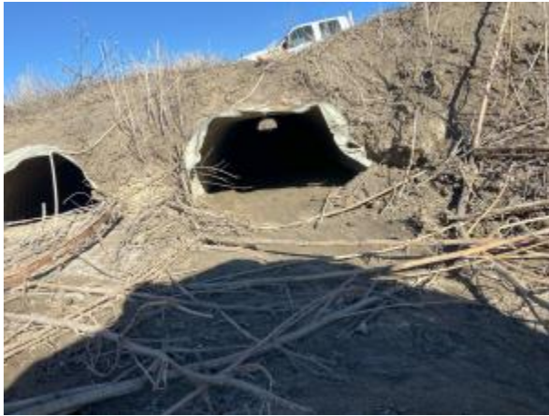
Photo No. 22, 12.03.2024 Observations
